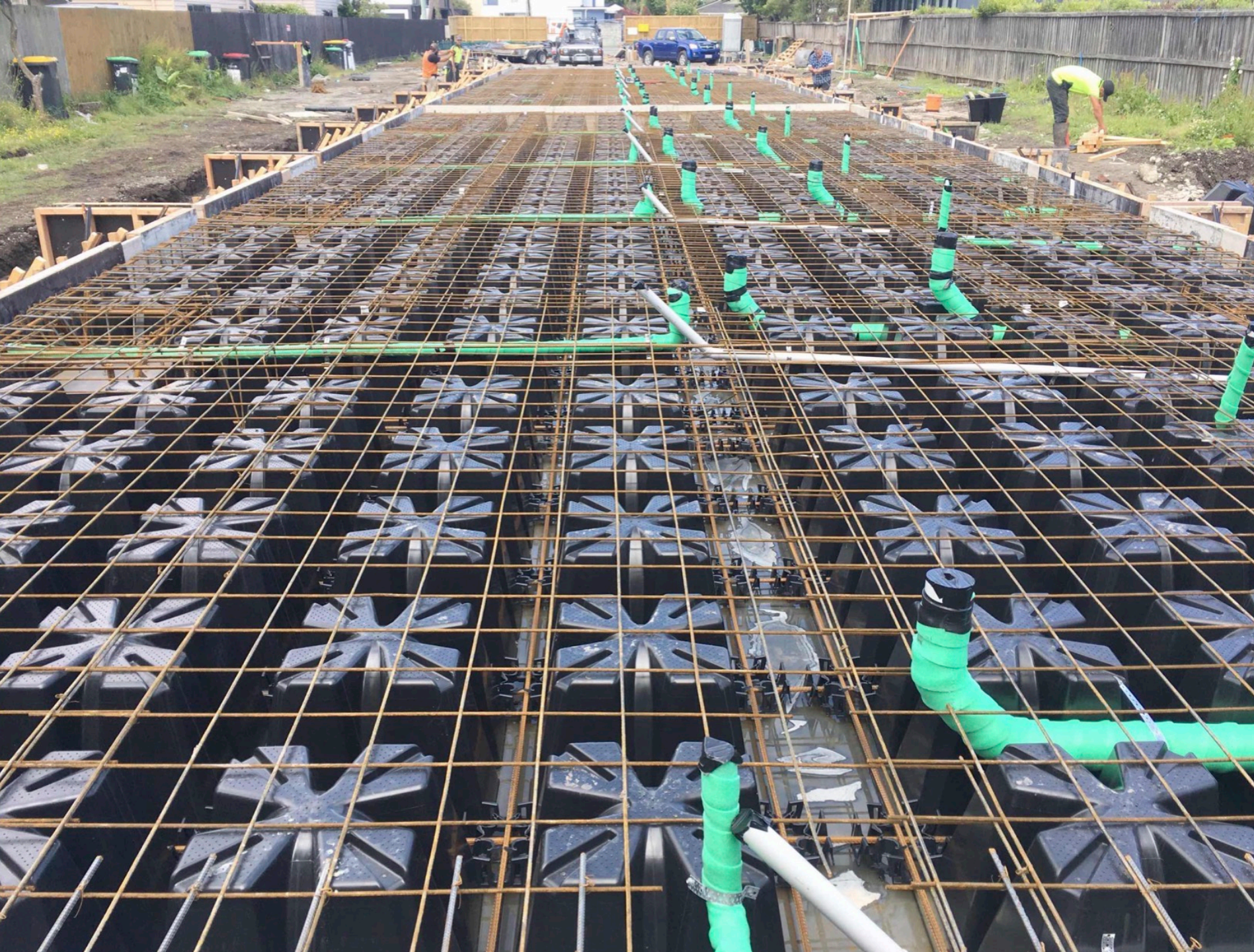
Drainage runs within the slab for future-proof performance and high efficiency on site.
